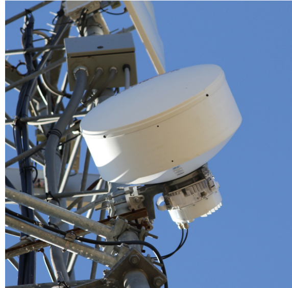
Solectek CM radio link installation at a major EMWD repeater facility near Winchester, CA
