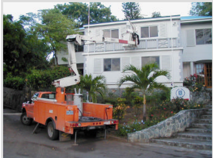
One of the last-mile radios is being installed at the Governor's mansion in the capital city of Roadtown.
