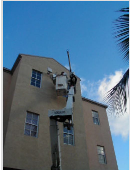
Solectek systems engineers are installing the radio and antenna on a rooftop and a wall. Mounting locations were determined in close consultation with the Government staff.
