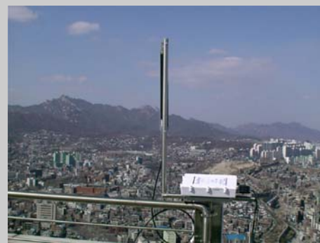
Installation of a SkyWay base station on a 34-story rooftop with a clear LOS in all directions
